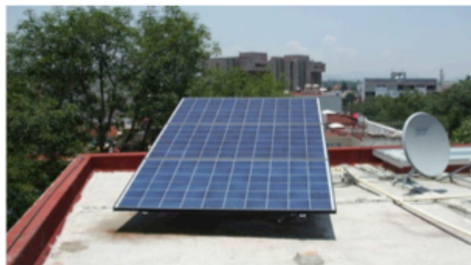
Lomas de Chapultepec, CDMX: 3+3=6 módulos, 2.5 kWp – P4214/4944
