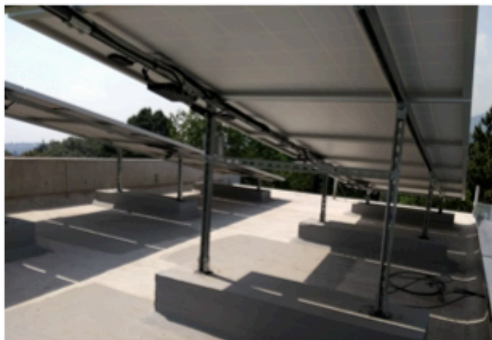
Contadero, CDMX: 24 módulos, 6.48 KWp – P4842
